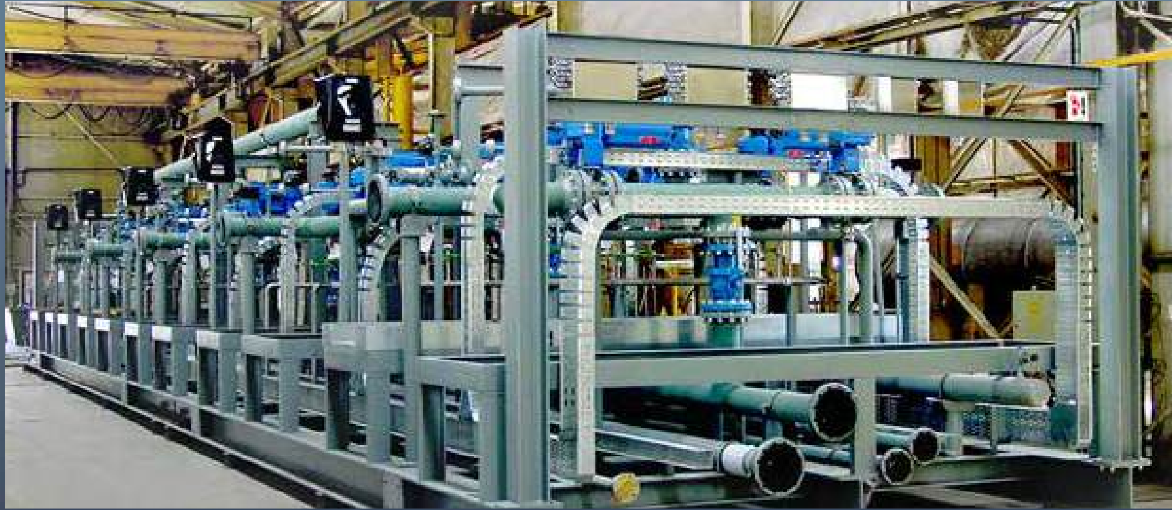
POLY BED HYDROGEN PURIFICATION SKID
